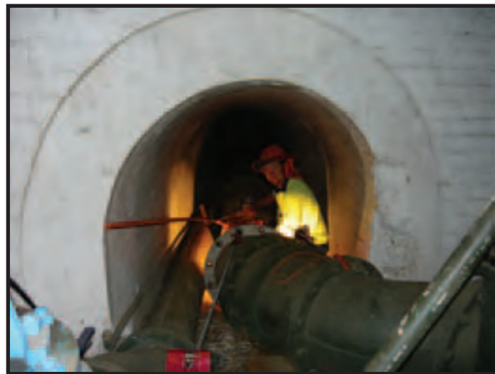
Riverina Water's Fitter Mechanic -Kane Cathro pulling stainless steel liner into river suction main
